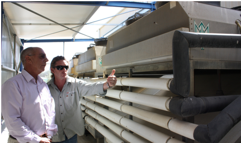
Gavin Colbourne, Production Manager at Phase Change Products Australia, explains the PCM thermal storage system to Jim
