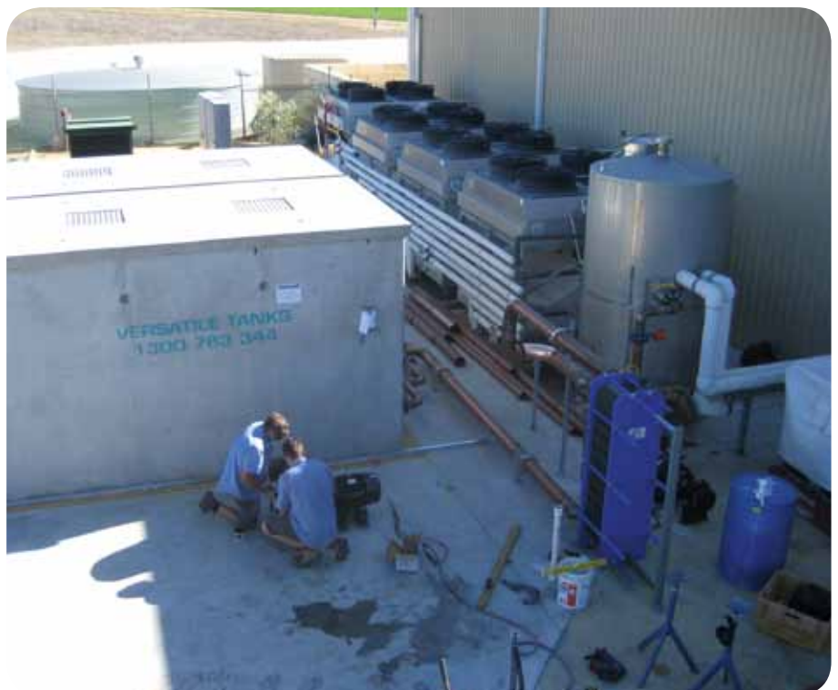
Phase-change material increased the farm’s cooling capacity without the need for extra chillers.
