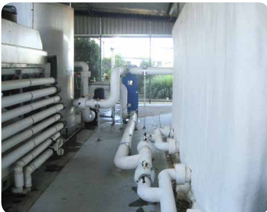
Chillers - thermal storage tank.
